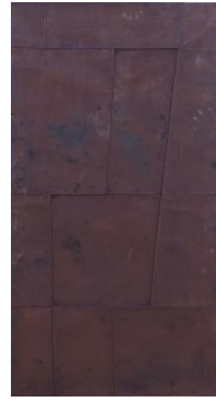
REAL RUST WREAKAGE
